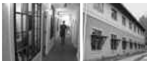
Large windows and savings glass panels allow natural light and create 90% of program space.
