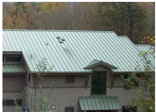
The steel roof is more effective at cooling than asphalt shingles, and the paint on the exterior is made with ceramic for better heat reflection.
