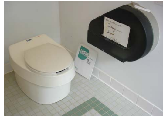
The Composting Toilet
