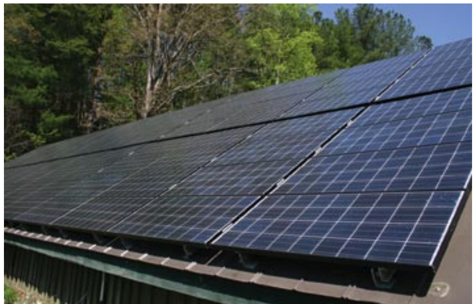
This solar array is used to charge the College’s fleet of carts, which are used by many work crews on campus. Excess energy created by the array is sent upstream and used by the local power company.
